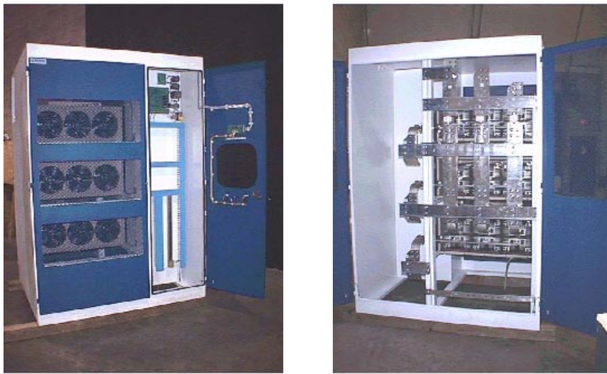
Figure 1. Front and rear views of the cycloconverter cabinet.
